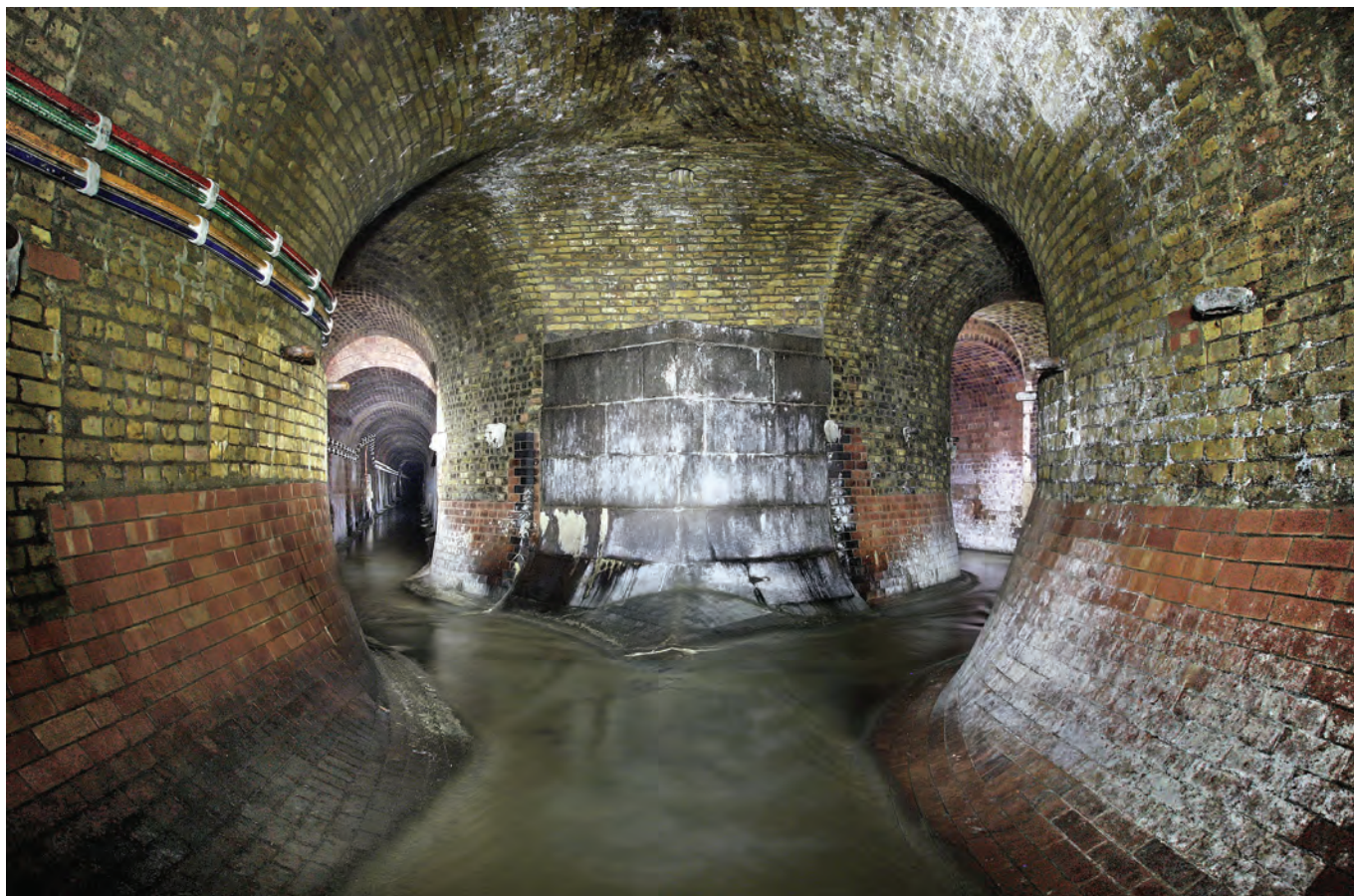
Possibly London’s most famous sewer intersection. The River Fleet splits at Farringdon Road and the two paths go their separate ways for a bit, rejoining just before reaching the Thames. Photo Adam Slater
